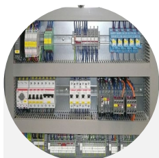
Sub- distributions flush-mounted
